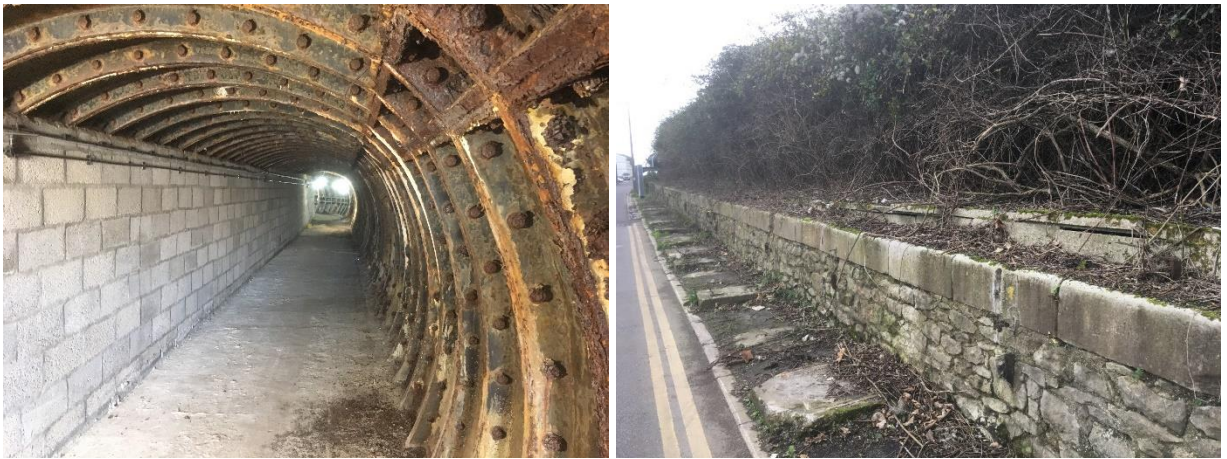
Plate 6 – a) tunnel adjacent to Incline Road; b) low wall and scrub adjacent to Incline Road/Main Road.
